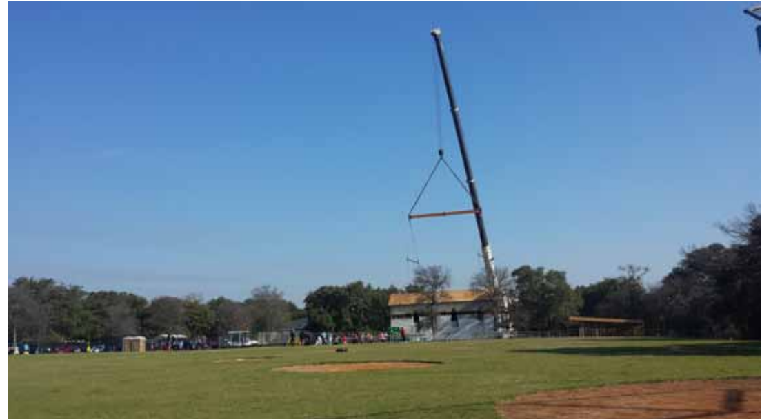
Moving an historic building from Brenham to Austin isn't easy. Here, workers in cranes and on the ground work to reset the roof on the building.
